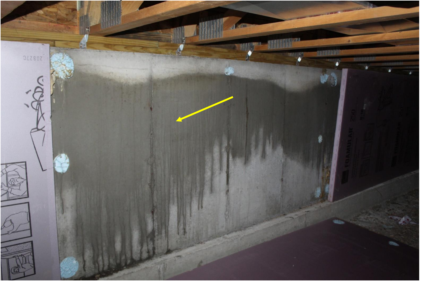
Water intrusion noticed in the crawlspace area. Soaked foundation walls noticed.
