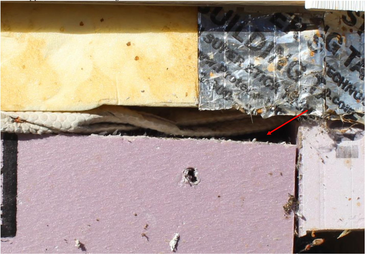
Water entry points noticed under the siding.
