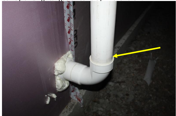
Some plumbing fittings did not have primer on them.
