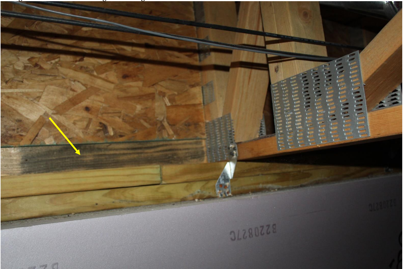
Mold growth on the wood framing & sheathing noticed in several areas.
