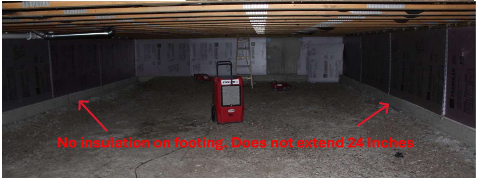
Insulation only goes to the top of the Footing
