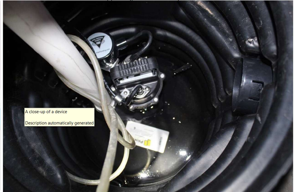
No holes were drilled into the bottom of the sump pit to let ground water into the pit.
