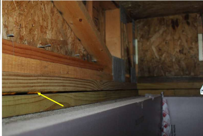
Poorly installed sill plates noticed.
