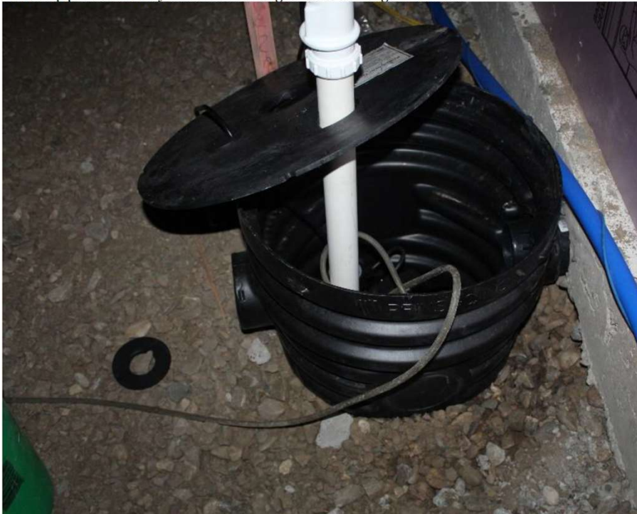
The sump pit was not fully installed into the ground to collect groundwater.
